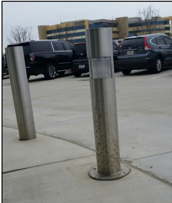
Stainless posts rusted from concrete finishing
