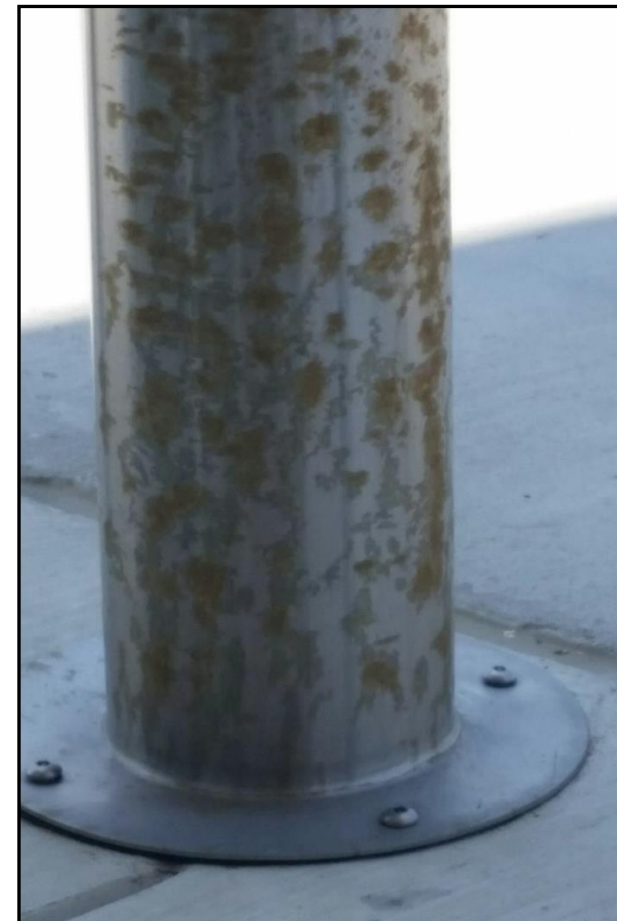
Close-up showing stains progressing
