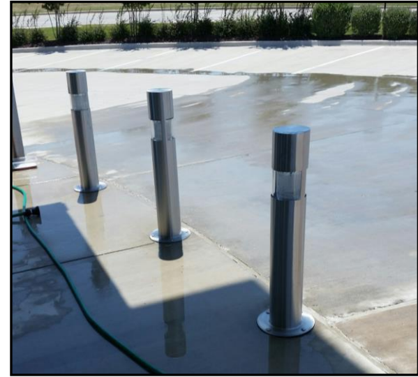
Center safety light posts (bollards) cleaned and drying to be sealed with EcoSeal Fortify to prevent re-rusting.
